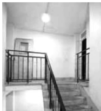
photo of stairwell with LED fitting
